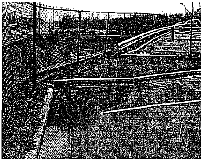
Figure 13. Settlement Observed Around SD6.
