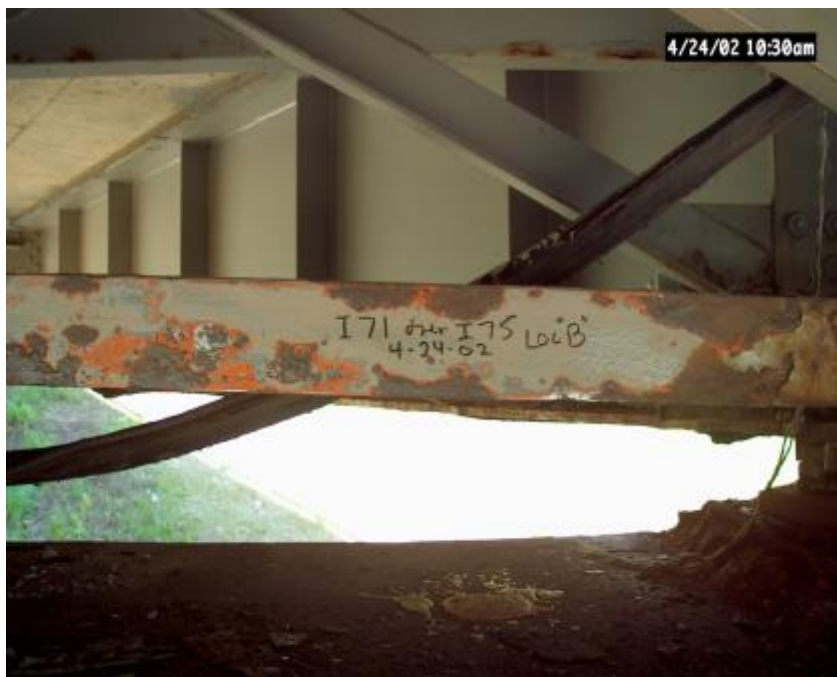
Figure 1 Detached Compression Seal Drooping Below a Deck Joint
