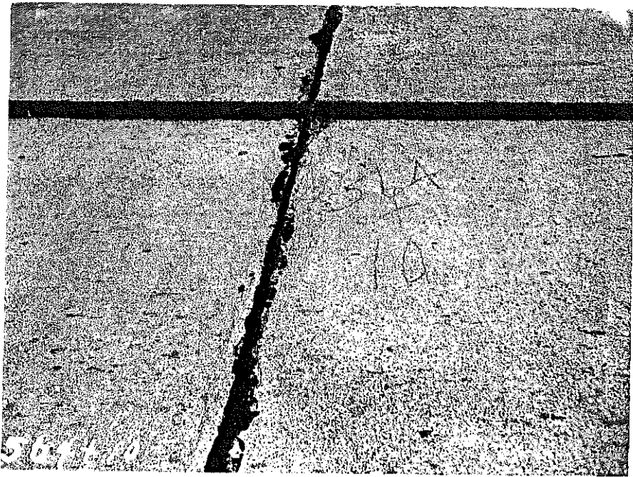
Fig. 5. Cracks formed parallel to a transverse joint at Sta. 564+10 on the Falmouth-Cynthiana Road. The coarse aggregate in this section of the road was glacial gravel, and the cement was normal portland. Only a few cracks parallel to joints were noted in 1947, but there was none in 1946.
