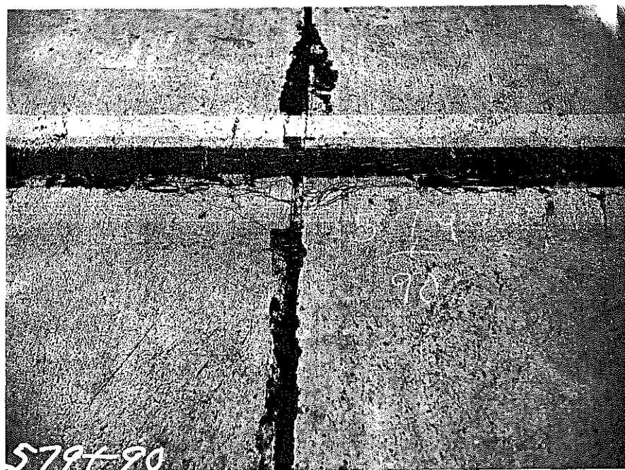
Fig. 4. A series of D cracks formed in adjacent slabs at Sta. 579+90 on the Falmouth-Cynthiana Road. The concrete contained a non air-entraining blended cement and gravel coarse aggregate. Several locations with cracks of this type that had developed during the past year are now evident in the two sections of concrete having gravel aggregate and no air entrainment.
