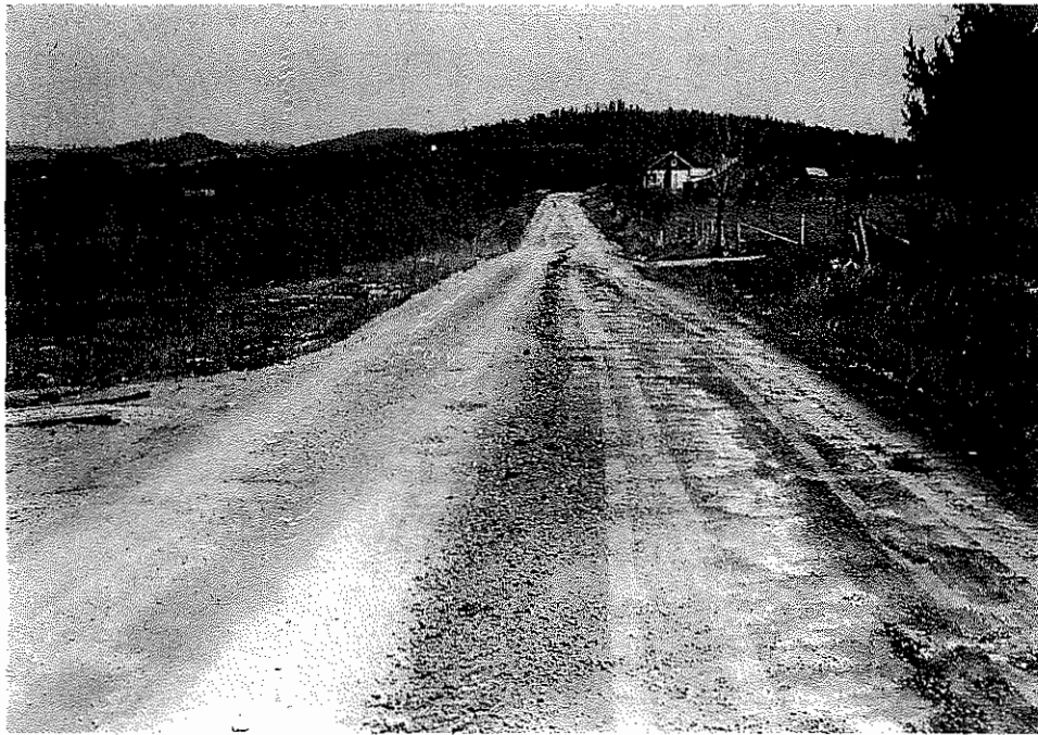
Fig. 16 - M.P. 100-855-E, Result of Absence of Crown, April, 1959.
