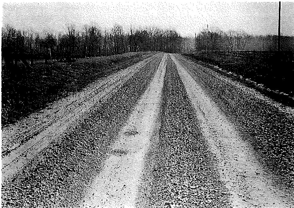
Fig. 18 - M.P. 069-450-B, Excessive Metal Which Can Not be Tied Down, April, 1959.
