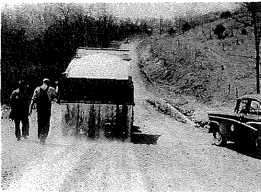
Fig. 11 - Gibbs Spreader in Operation, Uneven Application.
