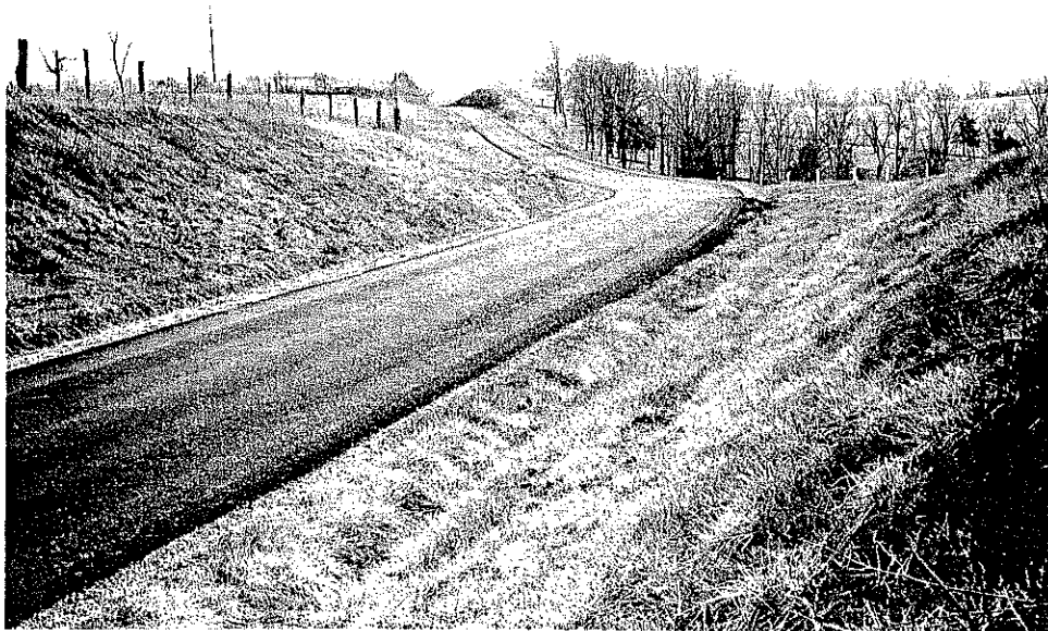
Fig. 4. Photograph Showing Area of Distress in Outside Wheel Track.
