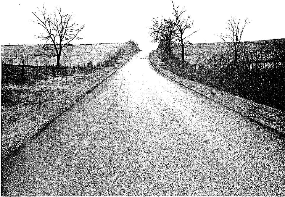
Fig. 3. Photograph Showing the Generally Excellent Condition of the Surface over the Entire Project. In the background are indications of some slight rutting in the right hand outside wheel track.
