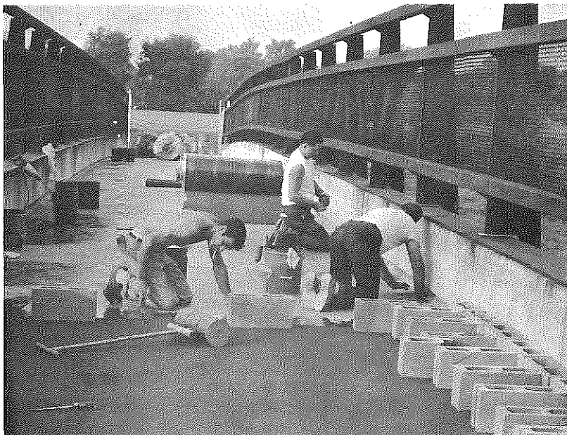
Figure 4. Anchoring Tartan Surfacing during Curing of the Mastic. Note Compression Roller in Foreground.
