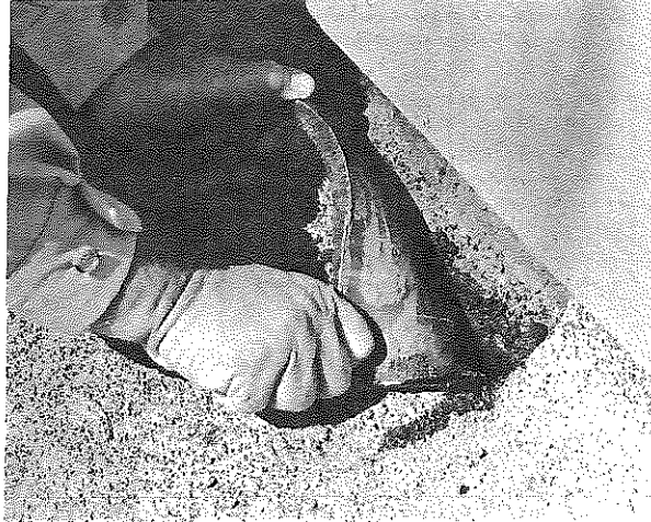
Figure 12. Unbonded Sheeting where Tucked into Raggle (4-25-73).
