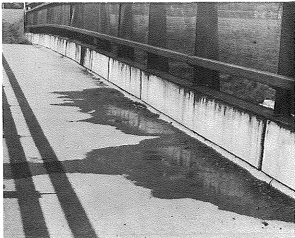
Figure 9. Standing Water near Middle of Span (4-25-73).
