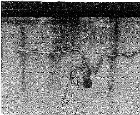
Figure 10. Crack in Concrete Plinth (4-25-73).
