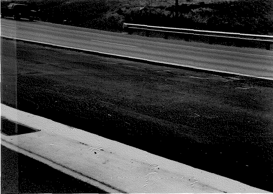
Figure 17. Median Drain Connected.
