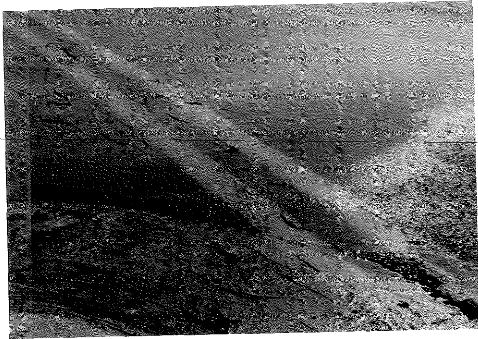
Figure 13. Water from Joint between Pavement and Gutter Wets Pavement.
