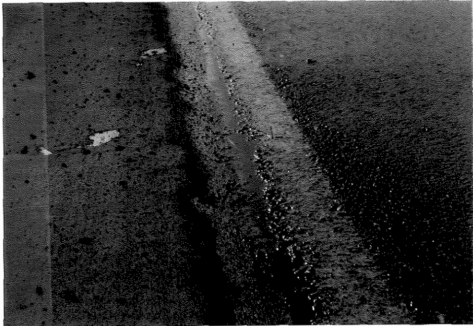
Figure 6. Close-up of Water Emerging, Northern End.
