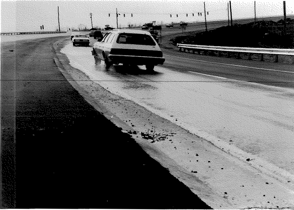
Figure 7. Water Emerging from Gutter Flows onto Pavement.
