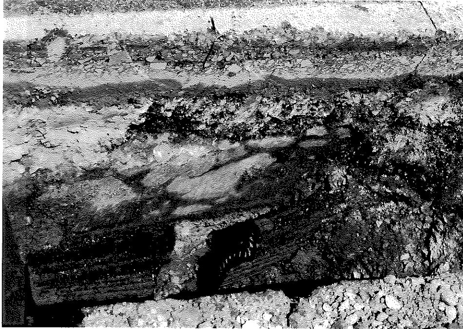
Photo 1. The top of the fabric "rolled over" and the support columns compressed on top of each other.
