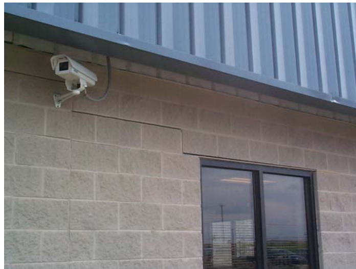
Figure 2.2. Crack in the Coalfields Regional Industrial Park office building (Karem et al., 2007).
