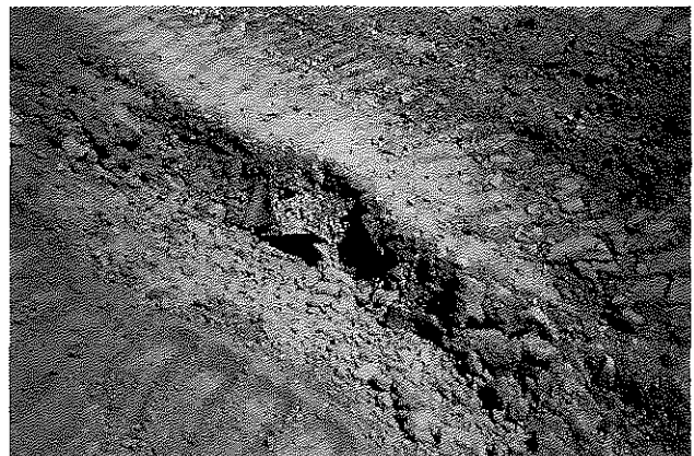
Figure 2. Top of cross drain damaged by pan at Station 531+15.
