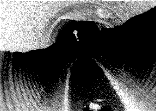
Figure 4. Damaged 30" cross drain at Station 619+00.
