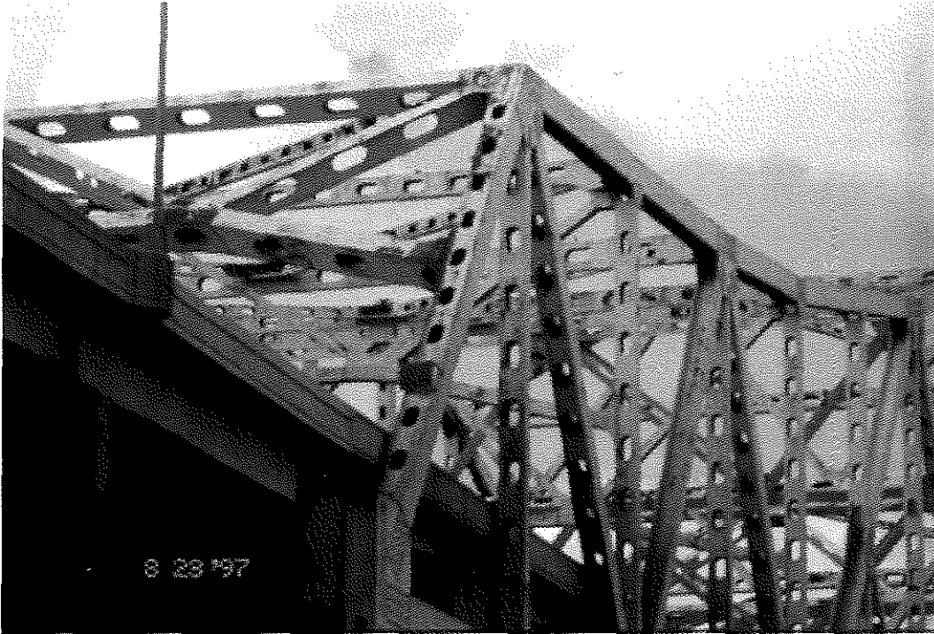
Figure 5. Close-up of Kennedy Bridge (note extensive rust in splash zone).
