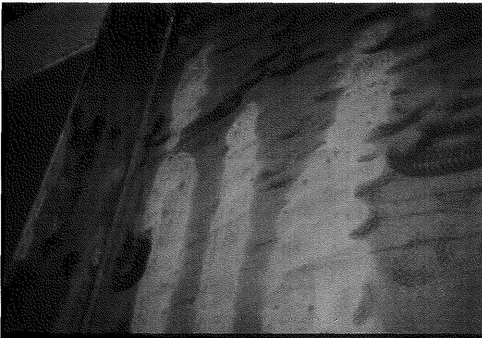
Figure 2. Water jetting removed the topcoat and much of the red lead primer.
