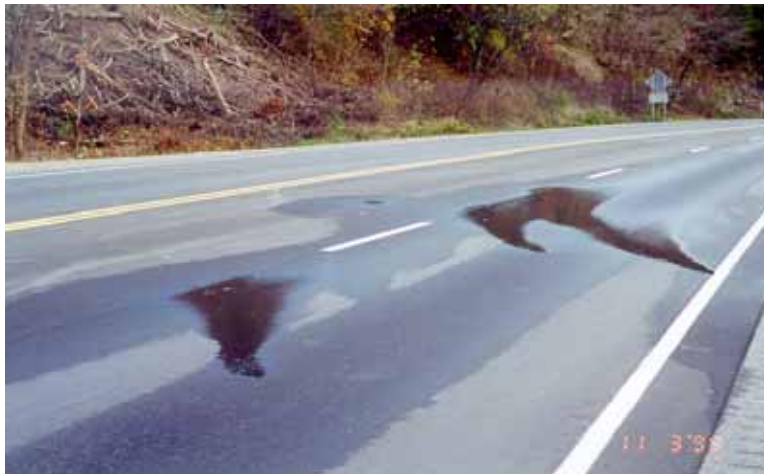
Figure 1. Water Coming Through an Asphalt Surface.
