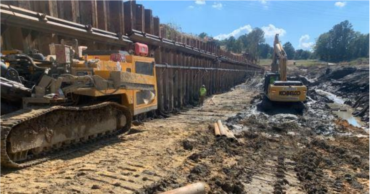
Figure 11. Earth retention system, 2021 anchor installation. Note the PVC pipe header attached to the wall connected to battered wellpoints installed through the wall face.
