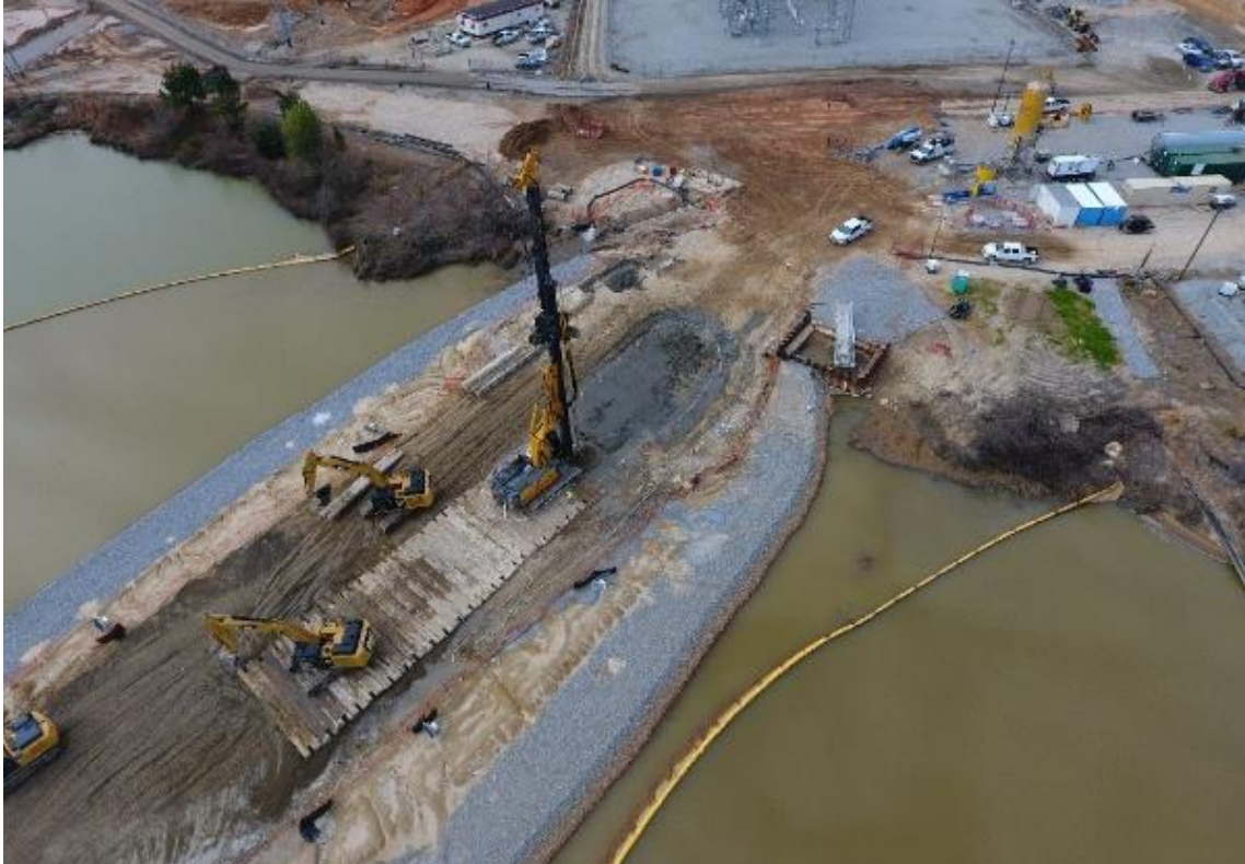
Figure 5. DSM operation on divider berm. Grout batch plant in upper right corner.
