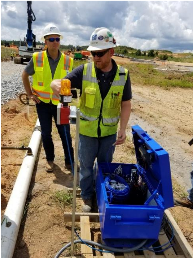
Figure 12. Installation of the geotechnical instrumentation system as part of the earth retention system.
