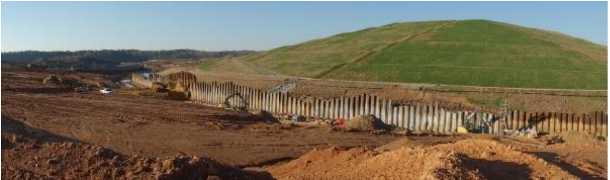
Figure 9. Panorama showing part of the earth retention system supporting the closed landfill.
