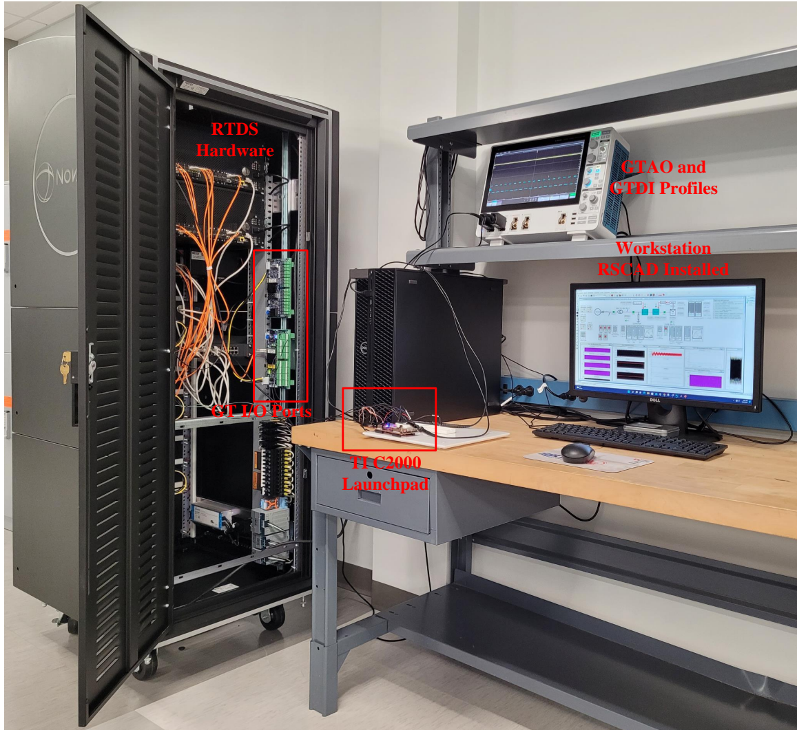
Figure 6.6: RTDS Control-Hardware-in-Loop experimental setup.
