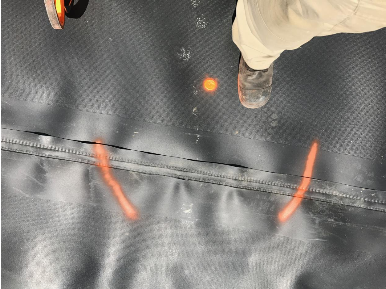
Figure 5. Excessive heat during fusion welding (entire seam, not just marked area).
