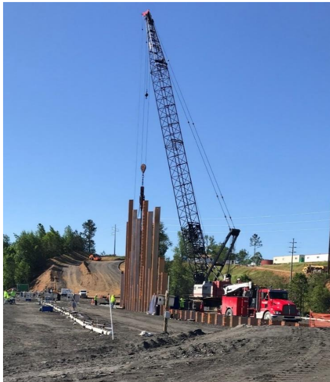
Figure 6. Sheetpile Installation. Note Dewatering Header on the Lower Left Side of the Photo.
