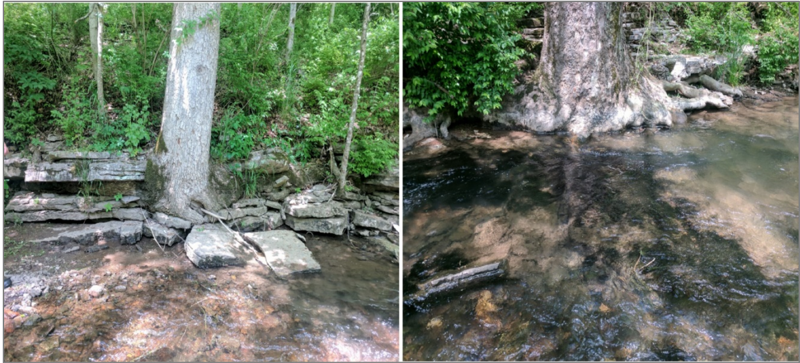
Figure 3.11: Block displacement mechanism by American sycamore ( P. occidentalis ) root penetration.
