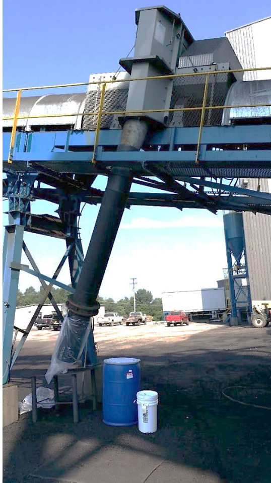
Figure 3.4. A sweep-belt sampler used to collect representative samples from the coarse refuse process stream of a coal preparation plant.
