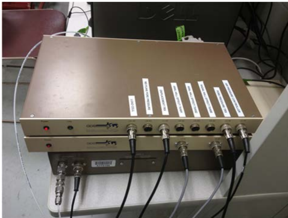
Figure C.26 Control boxes for unsaturated triaxial testing: (bottom) GDS pneumatic pressure controller, GDSPPC; (middle) bender element master control box; and (top) data acquisition 8 channel serial pad.
