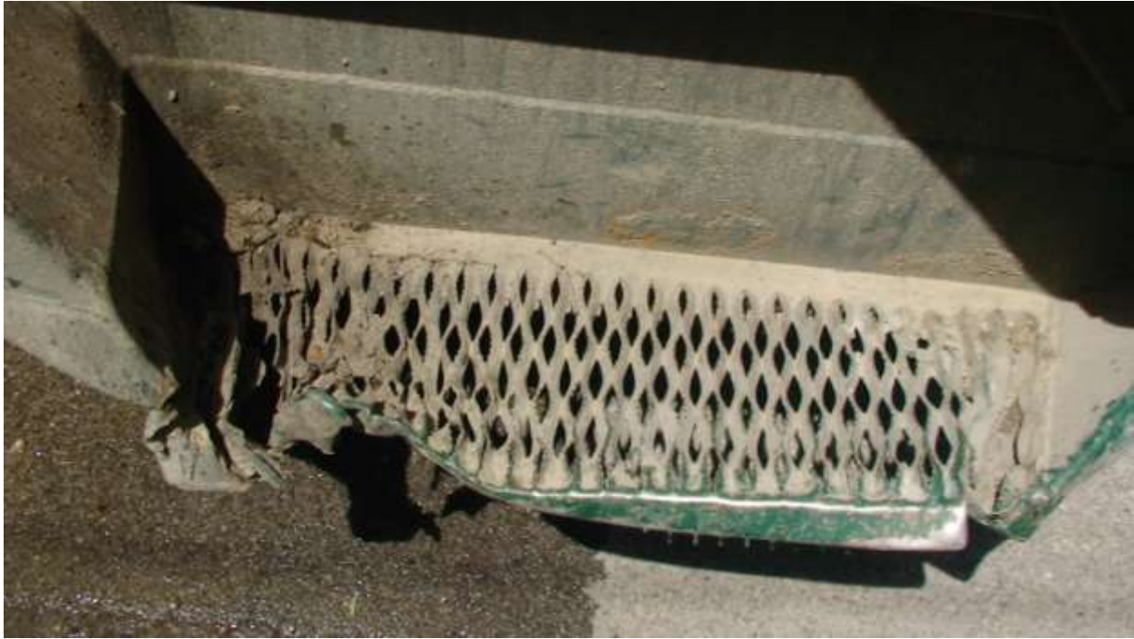
Photograph of broken step.. Photograph courtesy of KY Labor Cabinet.
