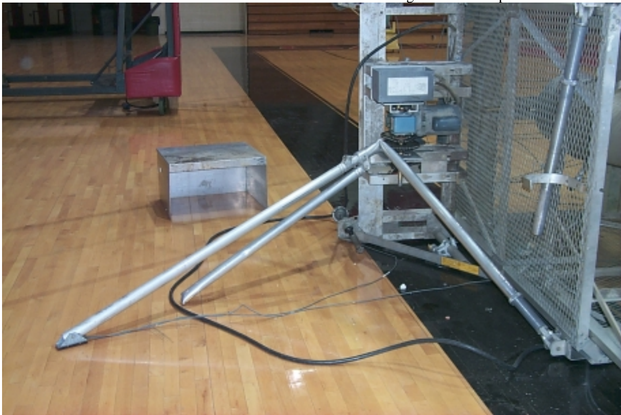
Picture of control ground control panel on its side and outrigger used to stabilize the lift. Notice it had been extended for use.
