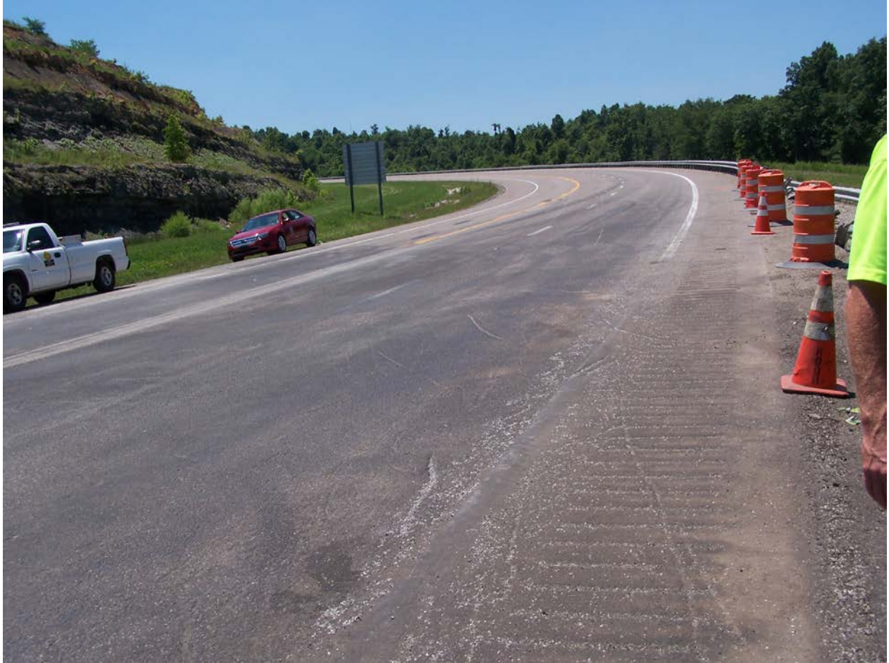
Photograph of state highway where incident occurred. Property of KY FACE.
