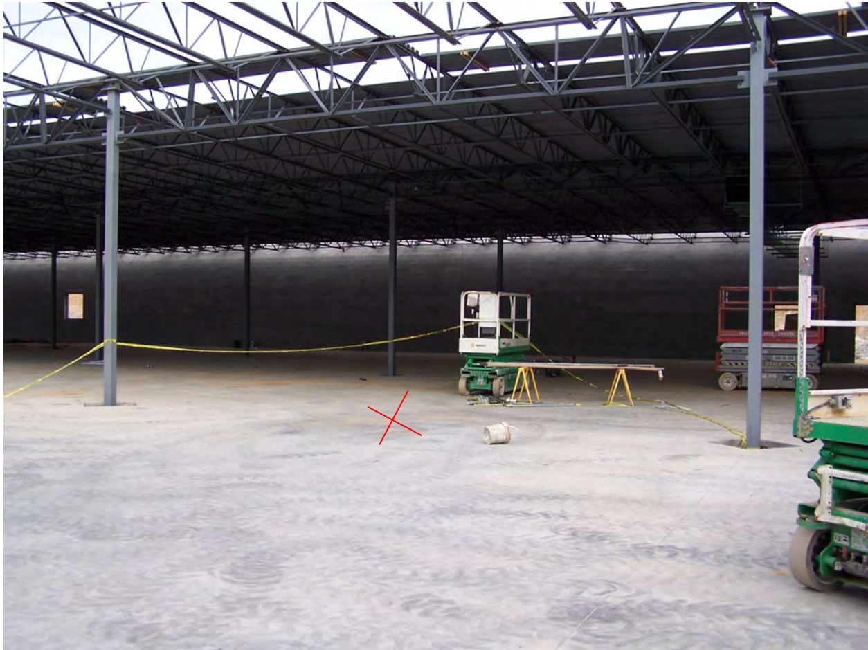
Location where foreman fell.
