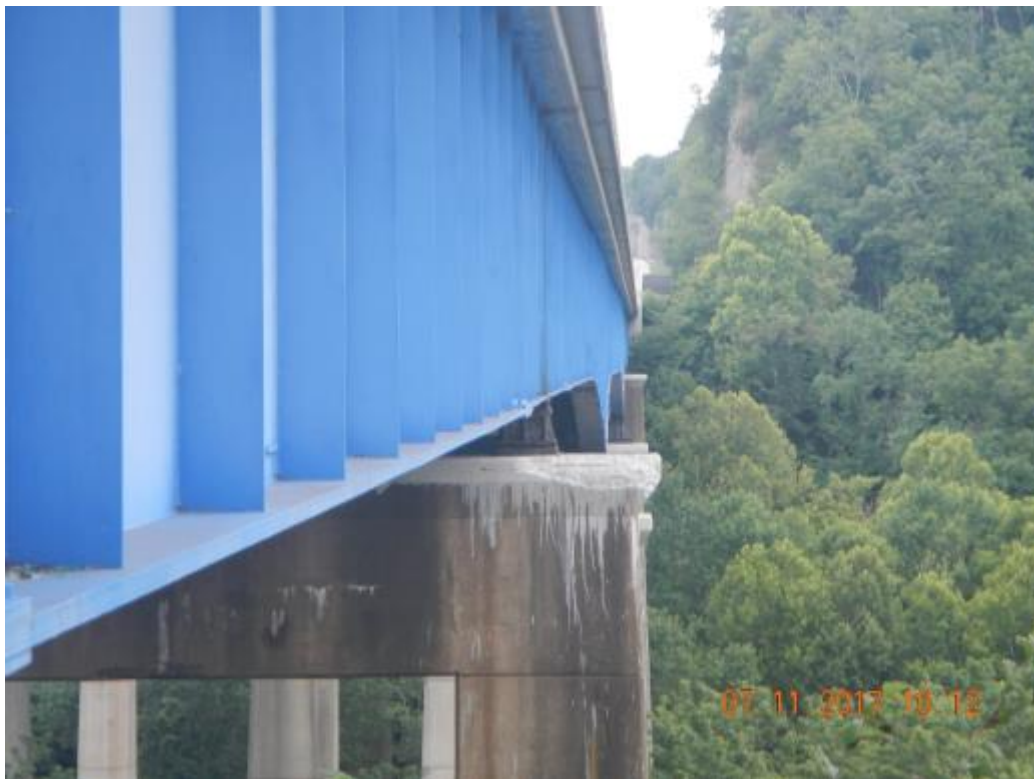
Figure 14 Severe runs — poor workmanship
