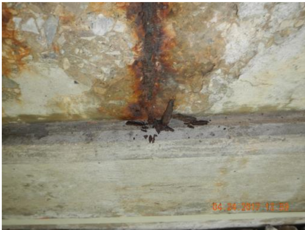
Figure 6 Loose rust after washing
