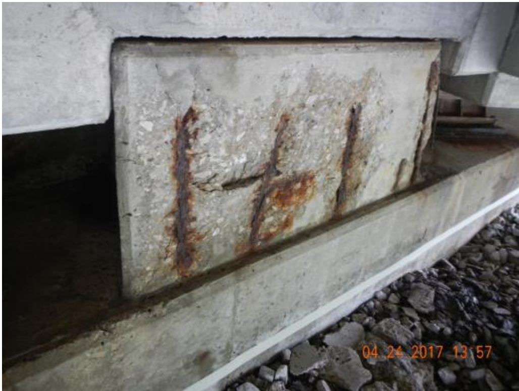
Figure 5 Spalled area on abutment after cleaning
