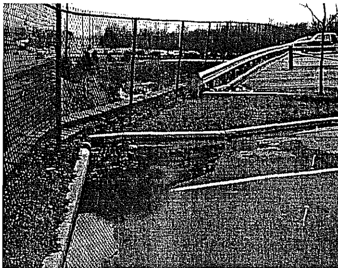
Figure 13. Settlement Observed Around SD6.
