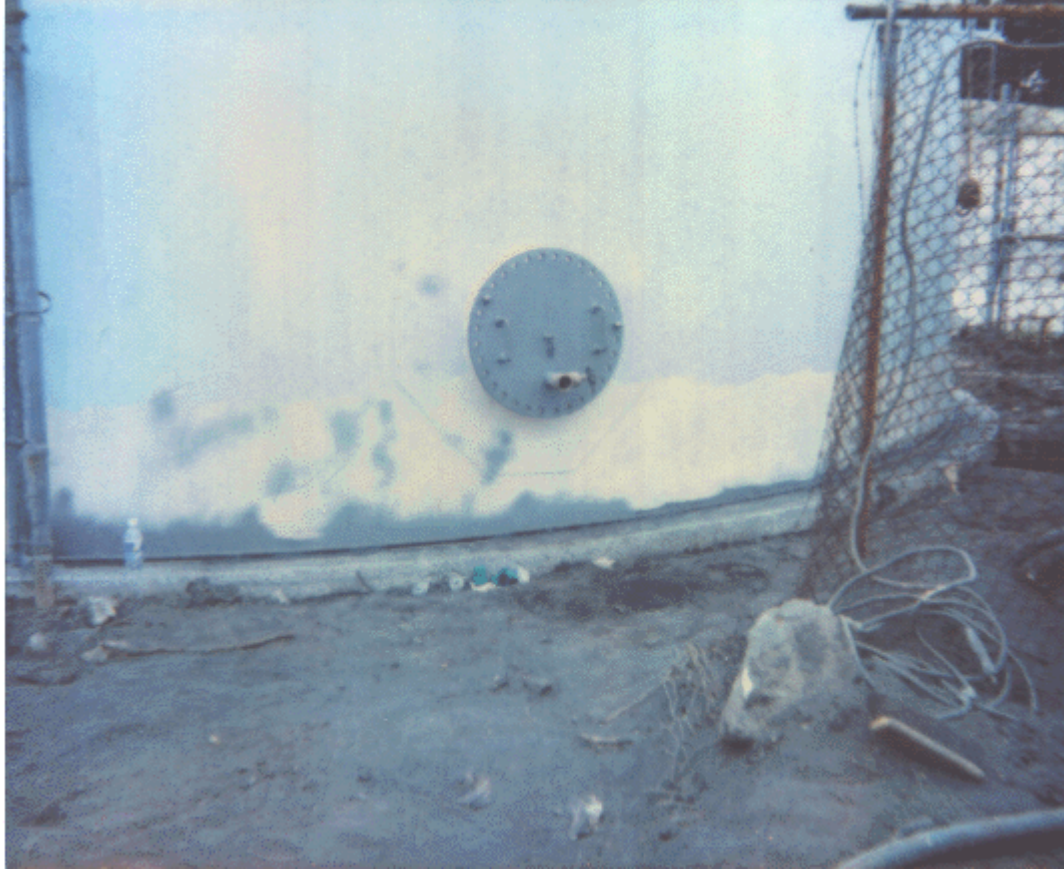
Picture of access / egress portal to water tank. The diameter of the access / egress is 24 inches and is 21 inches from the top of the concrete base, which is 5 inches deep.
